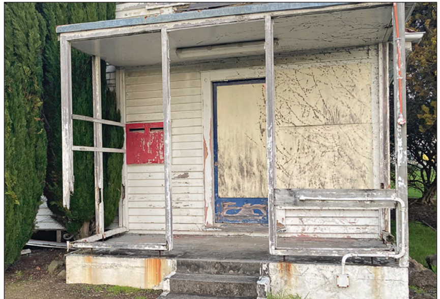
Dilapidated heritage... the former guardhouse at Fort Takapuna
