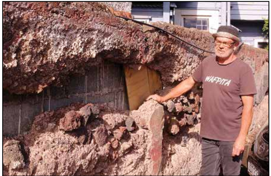
Crumbling heritage... Nicholas Philp is among neighbours who want Auckland Council to repair the Bear Garden Wall
